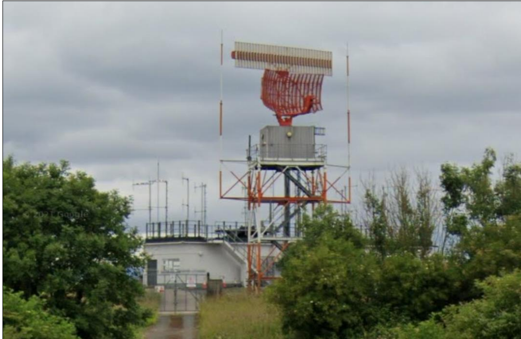
Figure 9. Dublin Airport MSSR Radar Station #1
