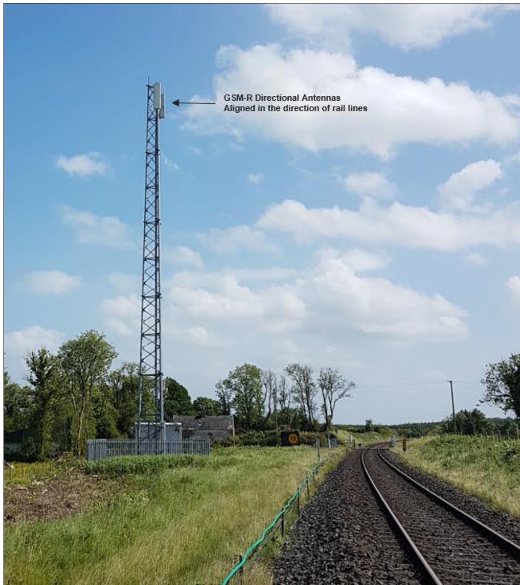
Figure 10. Example of a CIE GSM-R Basestation
